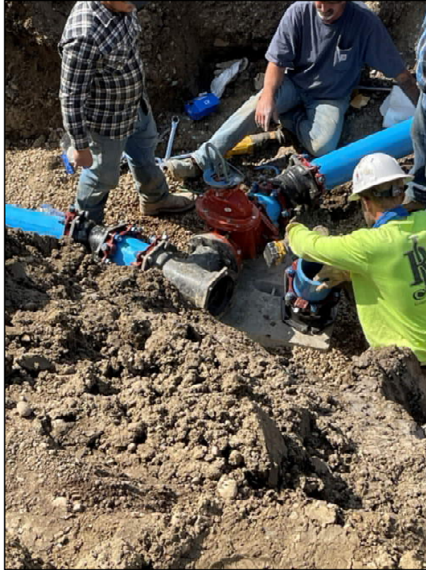
Figure 7: Installation of Gate Valve and Fittings – intersection of Hurly Drive and Perry Lane
