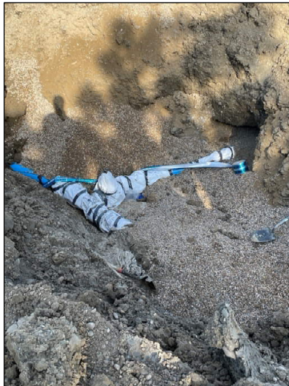
Figure 8: Wrapped Gate Valve and Fittings – intersection of Hurly Drive and Perry Lane
