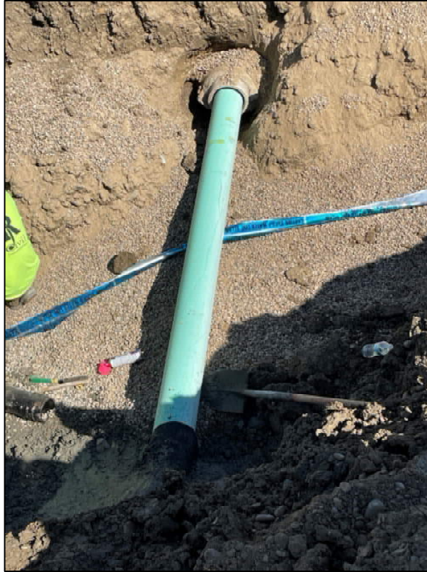
Figure 9: Damaged existing sewer main repair
